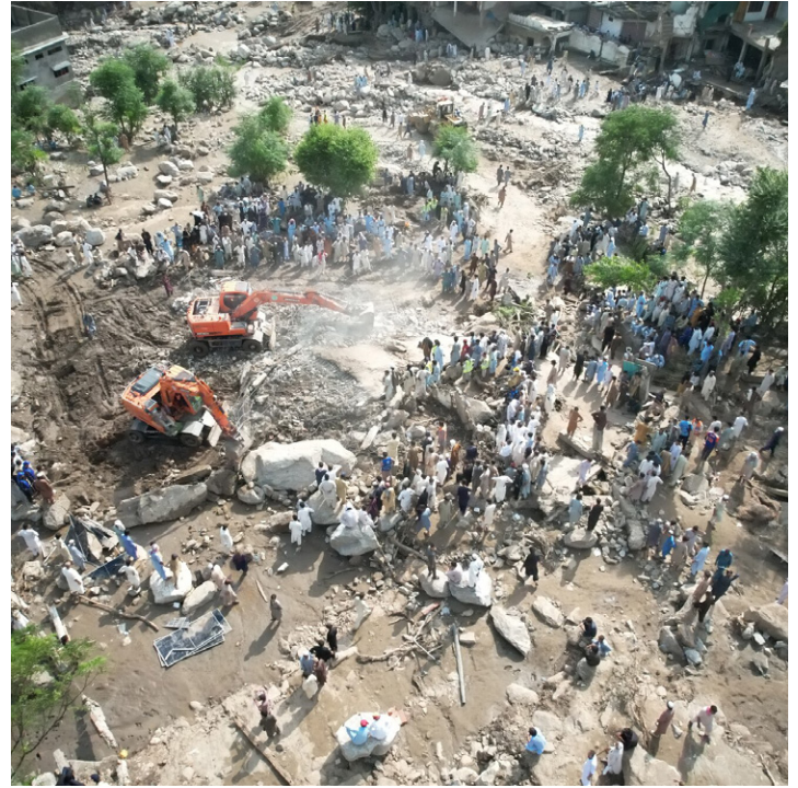
Swat, Pakistan, August 2025: Heavy flash flooding caused severe damage to homes, roads, infrastructure, and claimed precious lives
