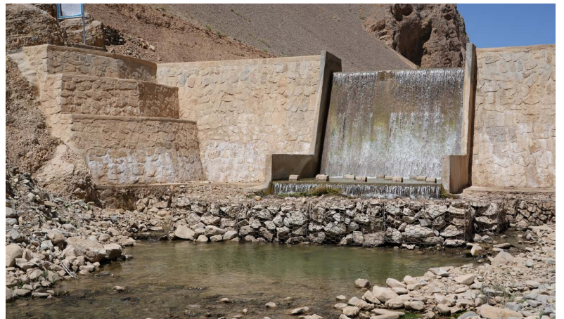
Constructing this 10,000 m3 capacity check dam in Ghor province has been crucial in preventing downstream flooding and making more water available for agriculture
