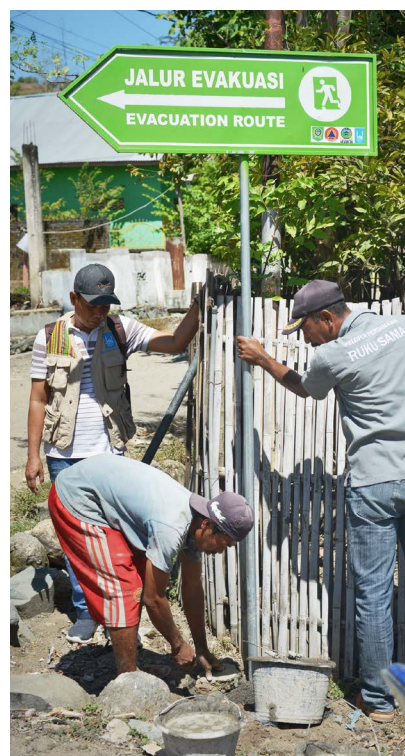
Erection of evacuation signage as part of the disaster risk reduction component of Islamic Relief's triple nexus programme in Indonesia [Photo: Islamic Relief, 2019]
